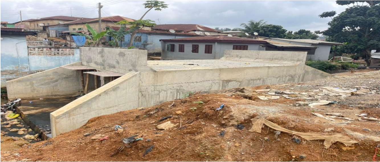
80% work completed on the construction of 2M x 2M double box culvert at Tutuka Tiatiaso.
